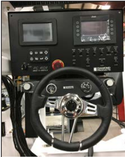
Centrally-located control station
